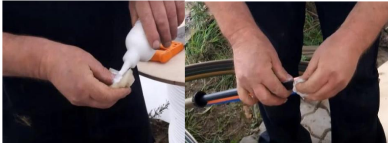
Fig. 4.25: (a) Sponge soaked with lubricant (b) Inserting soaked sponge into micro duct
