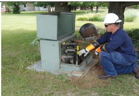
Fig. 1.20 Precautionary measures must be performed near the electric panel
