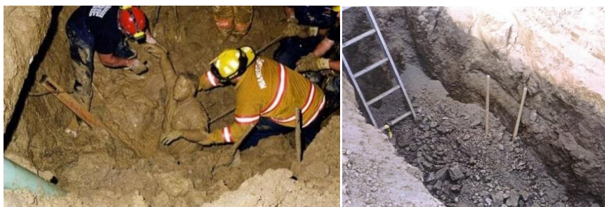
Fig.4.7 (a) Accident in the trench (b) Collapsing of the wall in the trench
