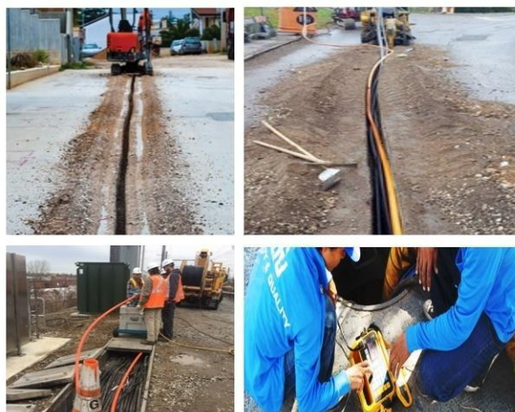
Fig. 1.10: Some task performed by optical fibre technician (a) Supervise the trenching (b) Perform ducting and placement of OFC (c) Technician performing splicing (d) Fault identification and maintaining the OFC
