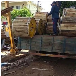
Fig. 2.4: Wrong way of unloading the cable drum by dropping it.
