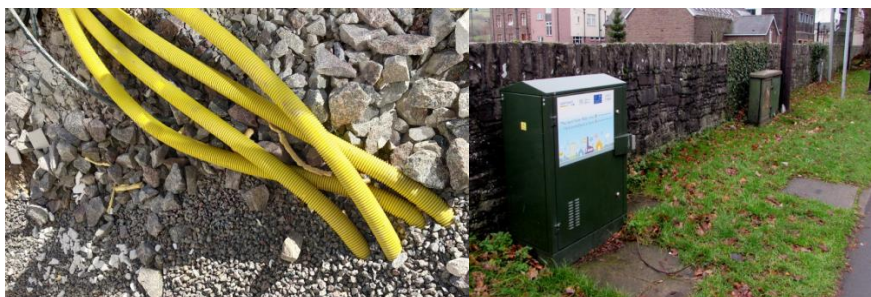
Fig. 1.5 (a) Underground cables (b) Telephone line junction box along the road
