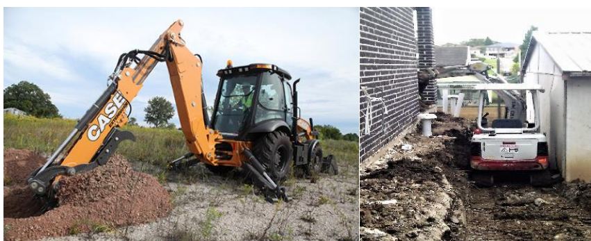
Fig.1.8: (a) Excavation in the open area (b) Excavation in the narrow area using a mini excavator
