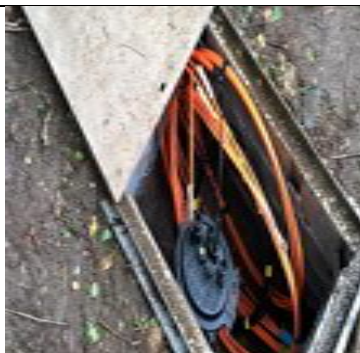
Fig. 4.21: Optical fibre cable kept in a manhole in the form of a coil
