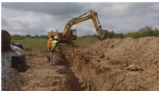
Fig. 4.4 Photo shooting Uneven trench width and depth
