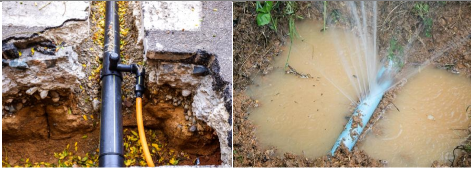
Fig. 1.9: (a) OFC close to water pipe (b) Water pipe damage in the excavation
