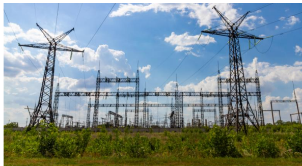
Fig. 1.19: Electrical substation and transmission tower
