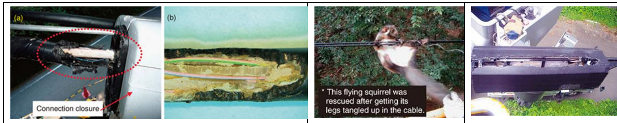
Fig. 1.13: Damage by a squirrel
